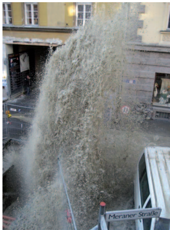
Pipe burst (cast iron, diameter 200mm) in Innsbruck, Austria. Credit: Innsbrucker Kommunalbetriebe.
